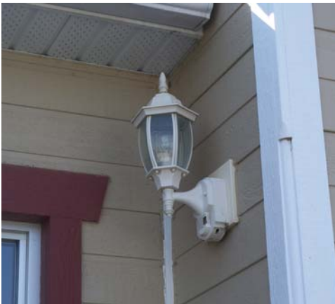
Prohibited decorative luminaire (Unshielded, exposed lamp)
