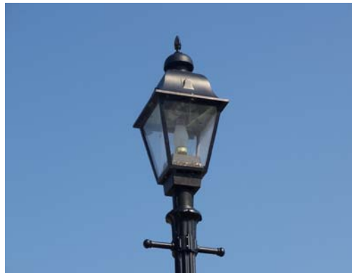
Prohibited pole-mounted luminaire
