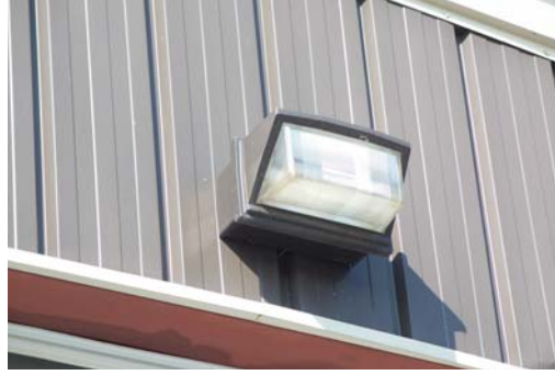
Prohibited wallpack luminaire
