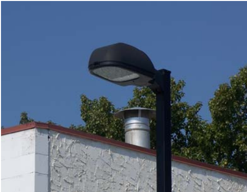
Permitted pole-mounted luminaire
